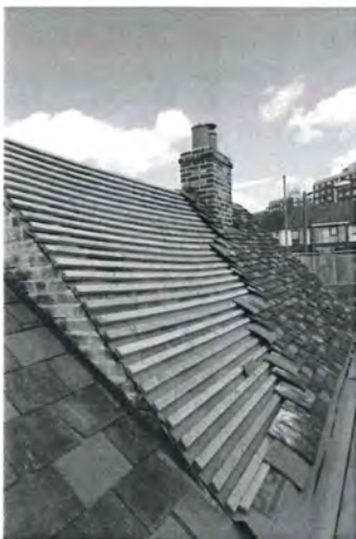
The clay tiled roof and chimney at number 22 in the course of repair
